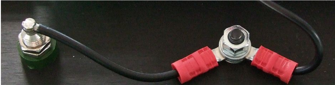
A 4mm banana socket is taken to the panel bond point which then is connected to the EPSU's 0VD or LINK terminal.
